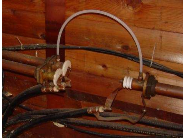
Figure 14.52: Flexible coaxial cables connected to rigid lines.
